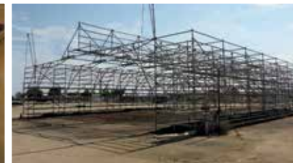
Large Qty of Scaffolding | Located in Bakersfield and will be sold by photo
